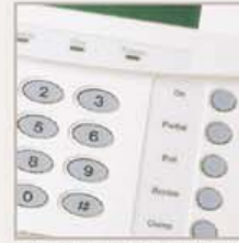
On, Partial, Exit, Bypass, Chime
